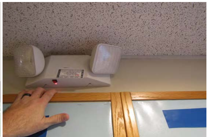
Emergency exit light did not function as designed
