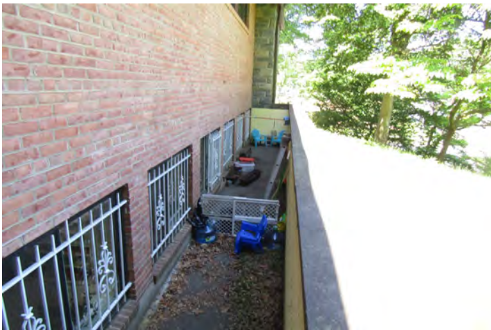
Debris buildup in the exit areas
