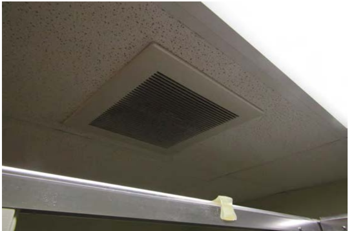
Debris buildup on the exhaust fan
