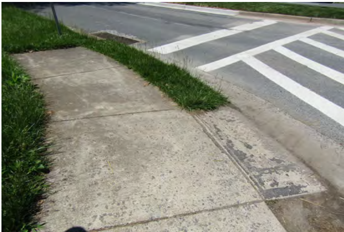
Runoff from the hill impacts city sidewalk
