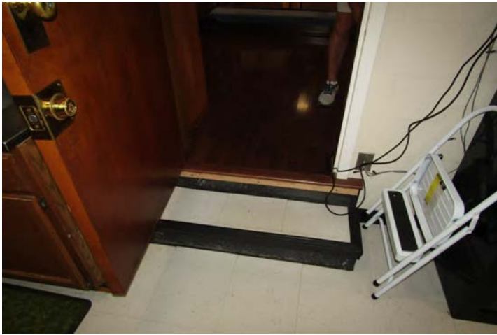
Access to sacristy needs a railing
