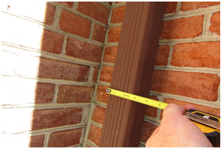
Downspout size is too small for volume
