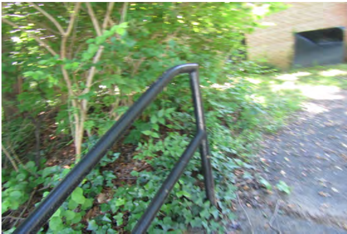
Handrail paint is chipped
