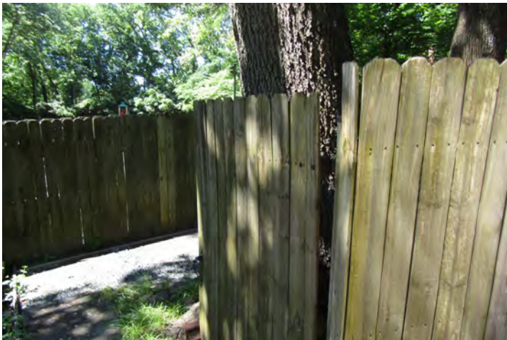
Fencing needs cleaning and resealing
