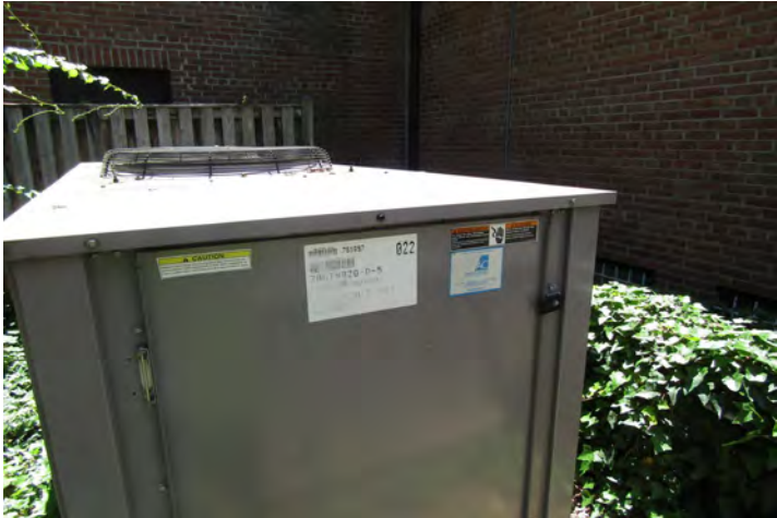
Chiller which shows landscaping being too close
