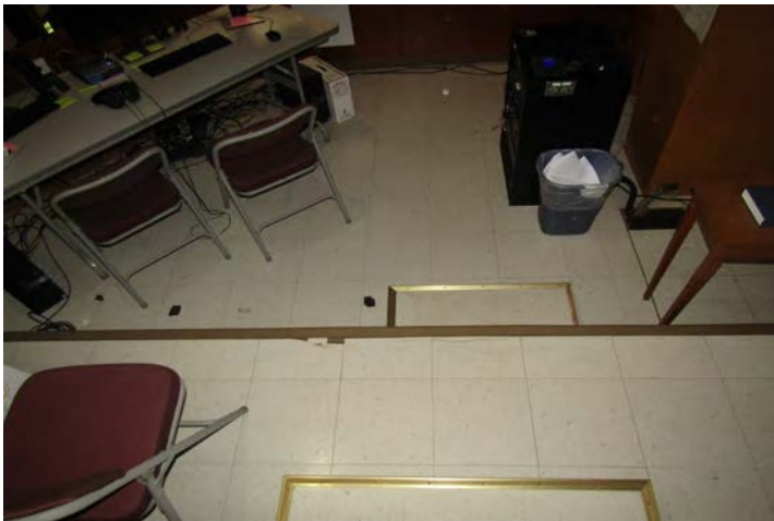
Potential trip and fall hazard
