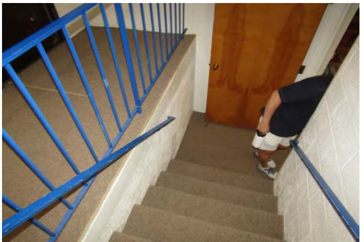
Musty smell indicates potential mildew in the stairwell
