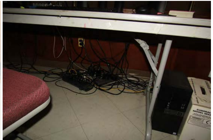
Cable management is poor
