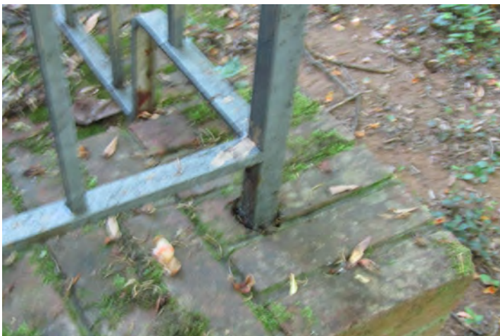
Handrail post base is damaged and missing grout
