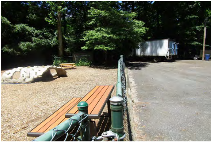
Playground fencing is crooked
