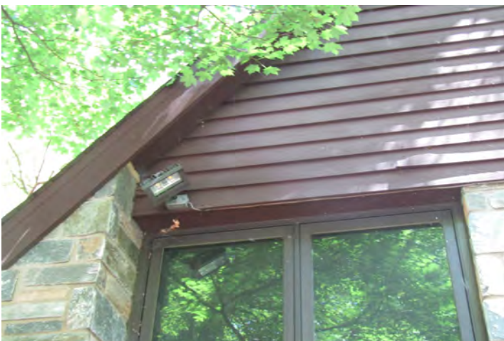
Siding has warped
