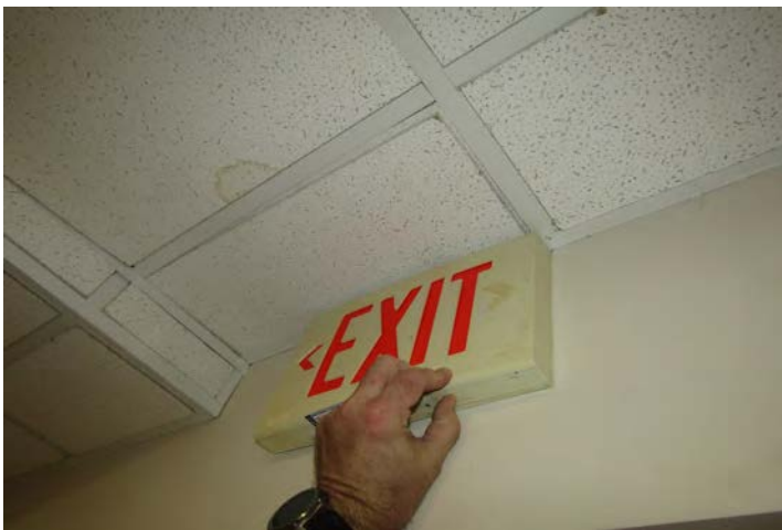
Emergency exit sign did not function as designed
