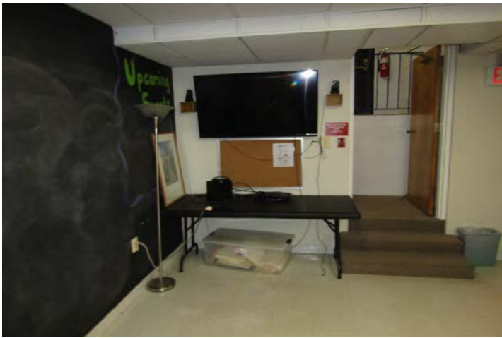
Access stairs need a handrail
