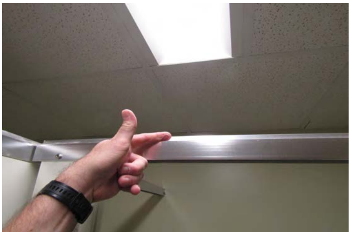
Debris buildup on the partition structure
