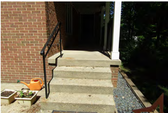
Stairs should have two handrails
