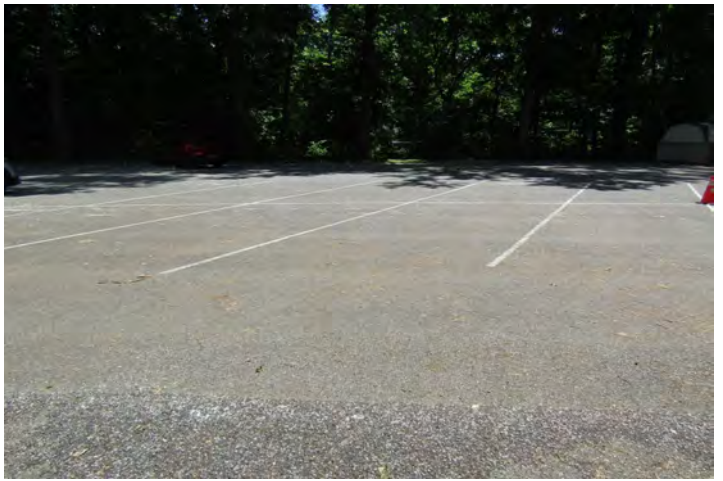
The parking lot seal and striping is faded
