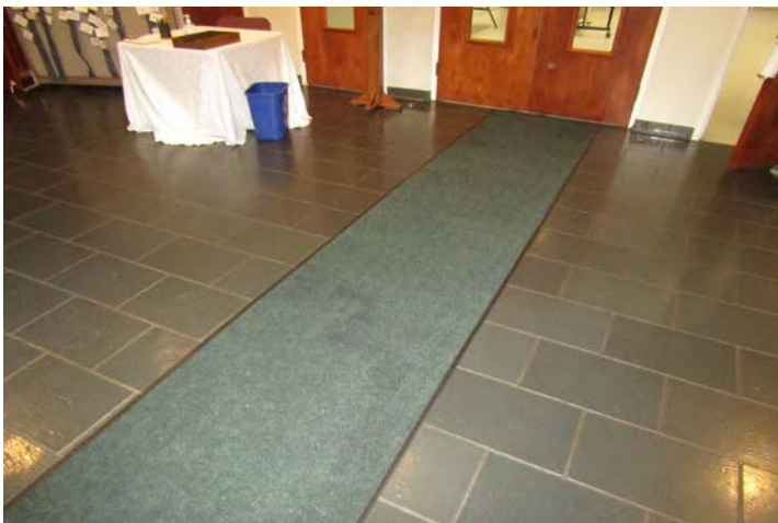
Entrance matting is worn and too narrow
