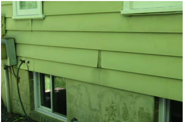
Minor areas of repair needed on the siding
