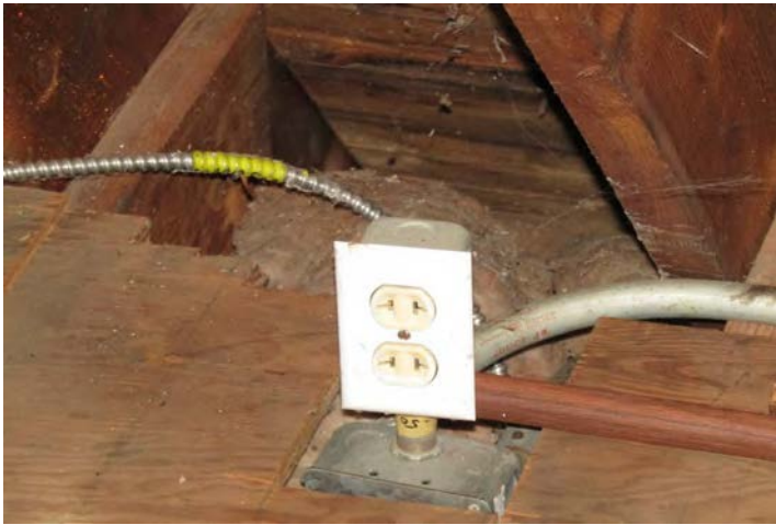
Ungrounded outlet, incorrect junction box for a floor mount
