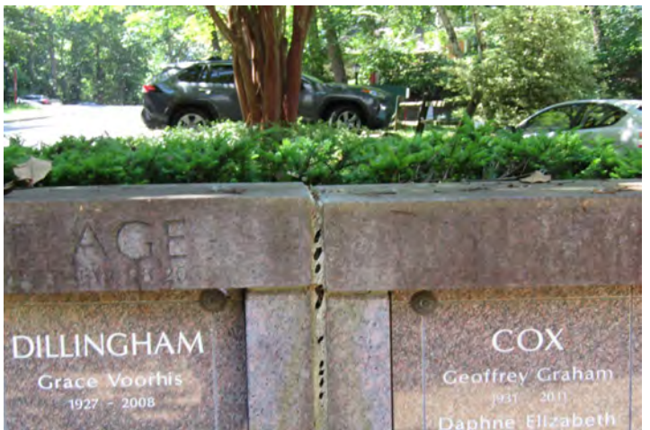
Shifting masonry or foundation at the Columbarium
