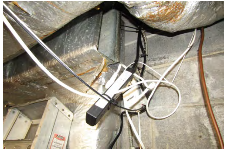
Suspended power strips and extension cords instead of proper circuits
