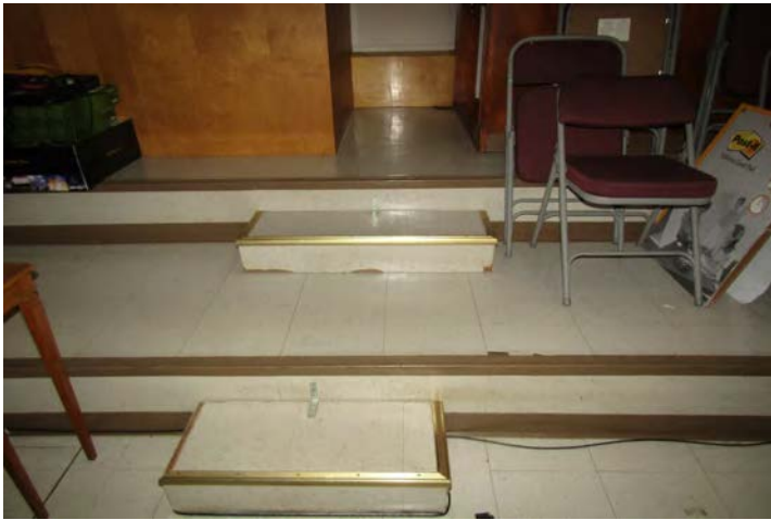
Steps need a handrail
