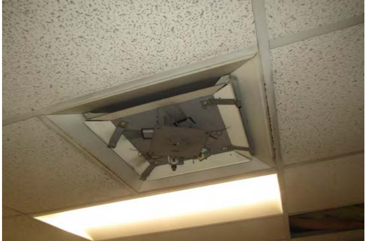
Broken HVAC supply vent
