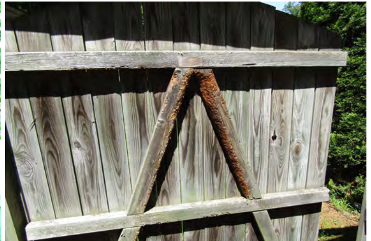
Wood damaged around the HVAC
