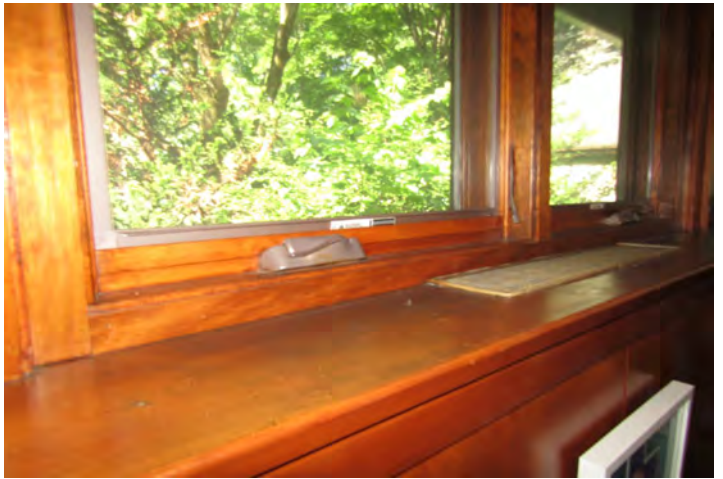
Wood needs cleaned and refreshed
