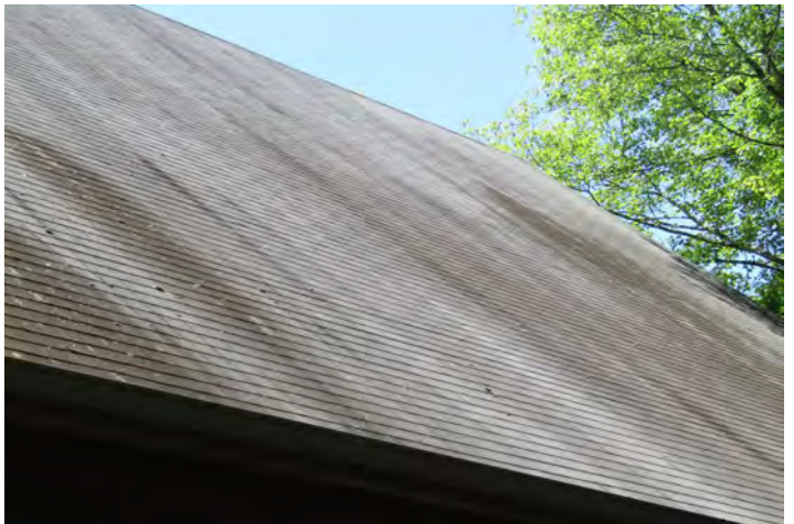
Shingles are past service life
