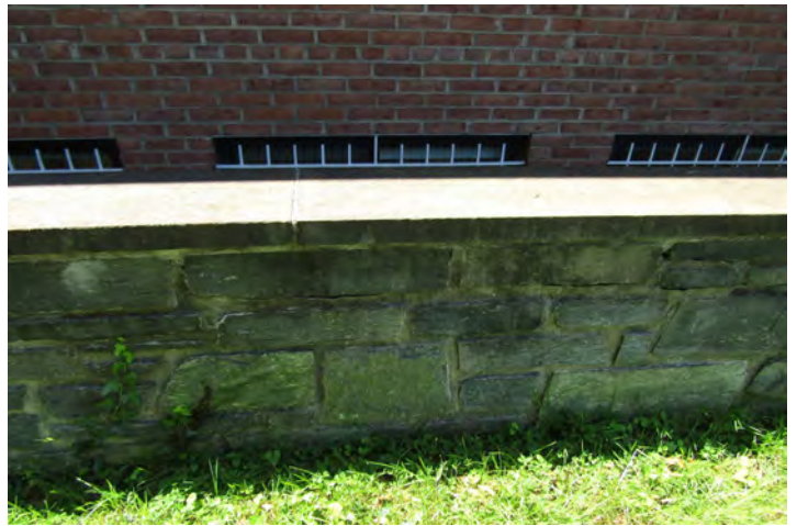
Masonry wall has shifted
