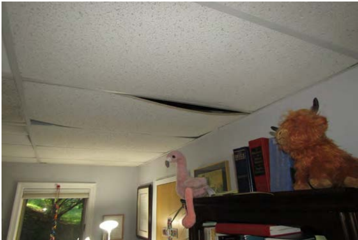
Ceiling tiles out of place
