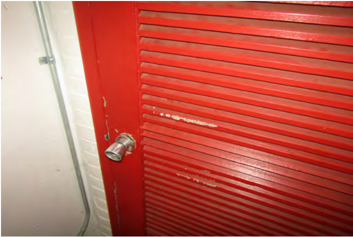
Chipped paint on the door
