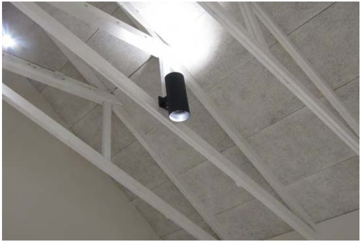
Cobwebs and debris on the light and framing
