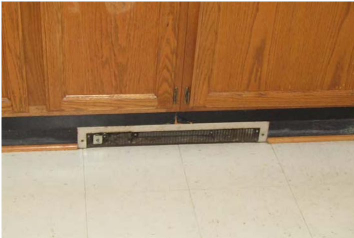
Debris buildup on the floor base
