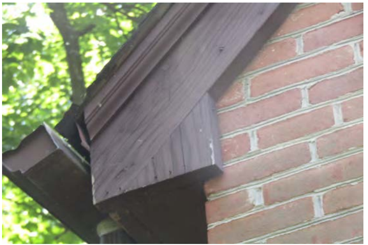
Damaged wood trim
