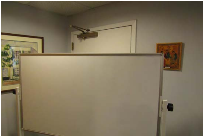
Egress door is blocked
