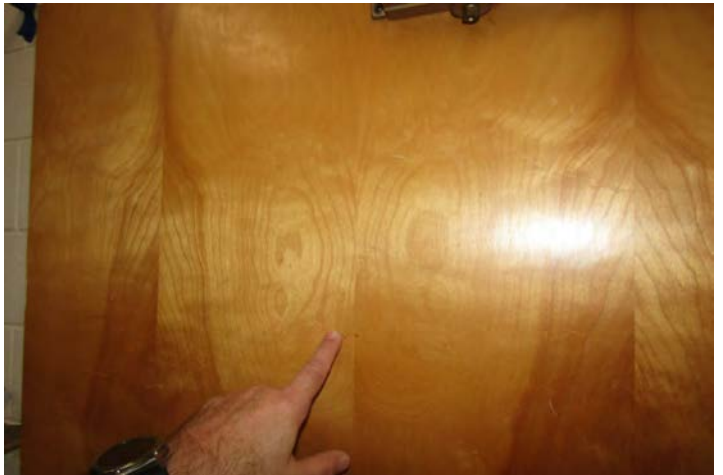
The door needs a door lite
