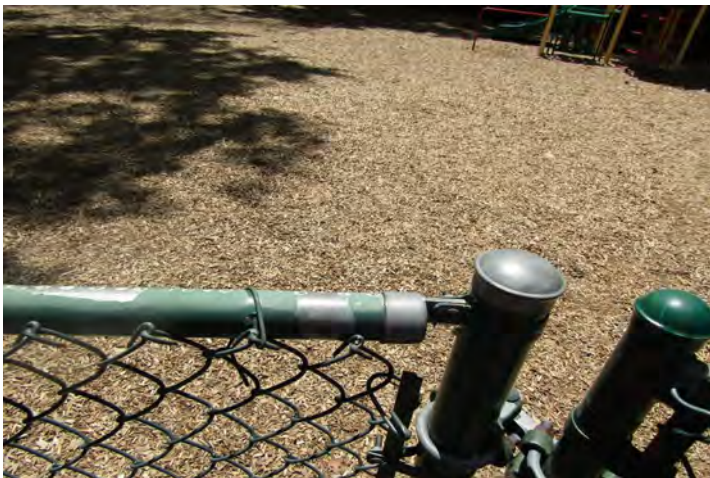
Chain-link fence paint is chipped
