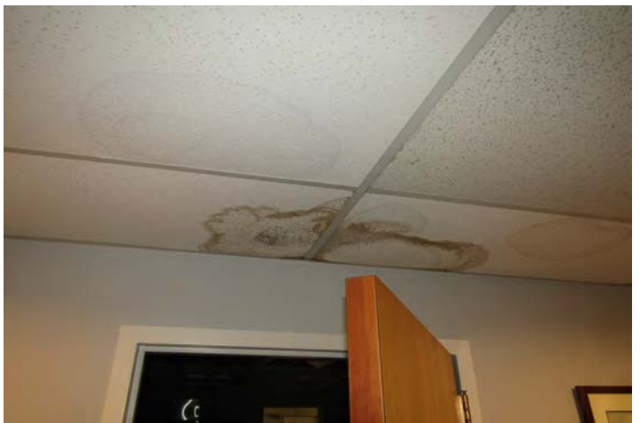
Stained ceiling tiles
