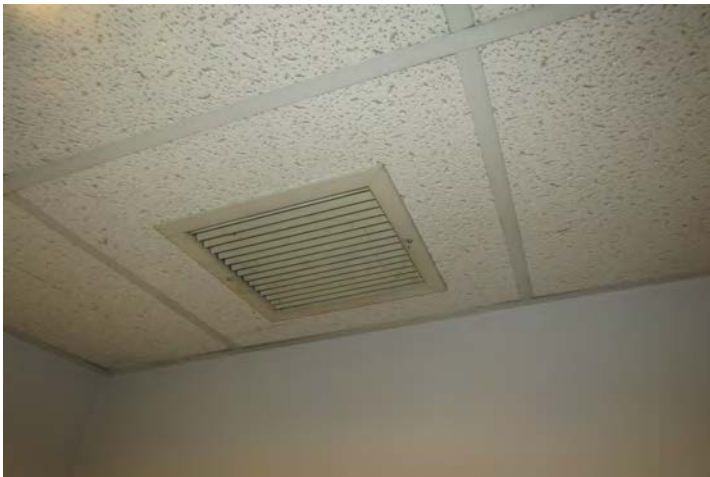
Debris buildup on the exhaust vent
