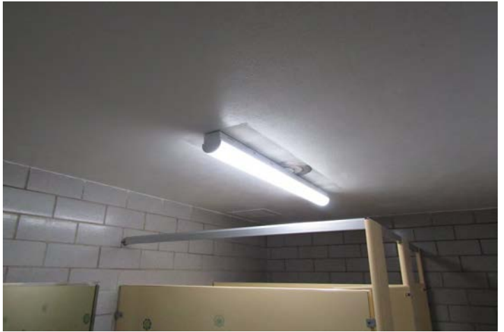
Ceiling touchup needed around the new light
