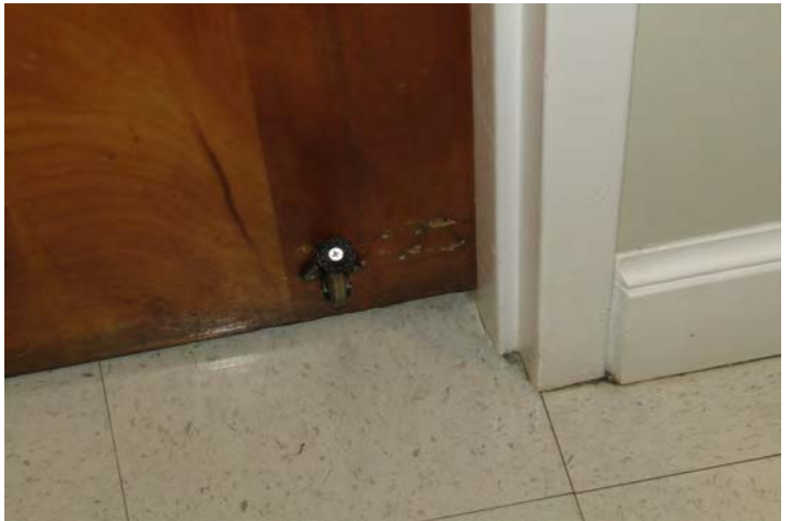
Door damage at the bottom
