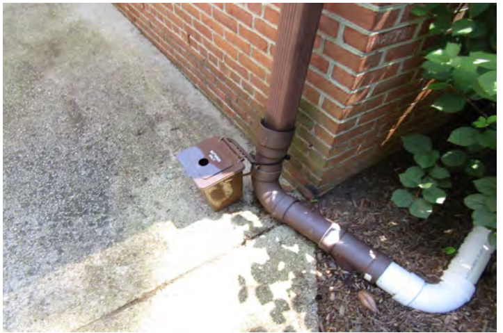
Drain has too sharp of a bend
