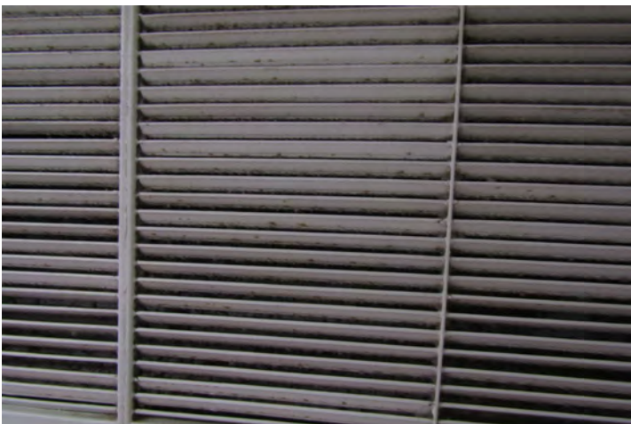
Debris buildup on the vent
