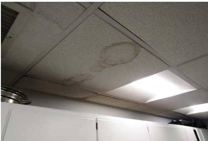
Stained ceiling tiles
