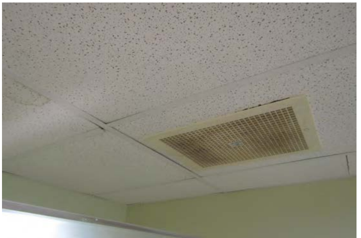
Debris buildup on the exhaust vent
