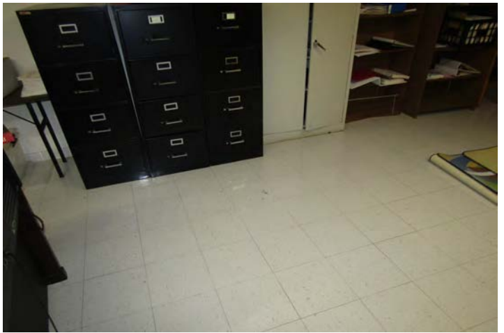
VCT floor needs a strip and re-wax
