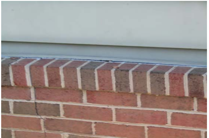
Caulking line has failed
