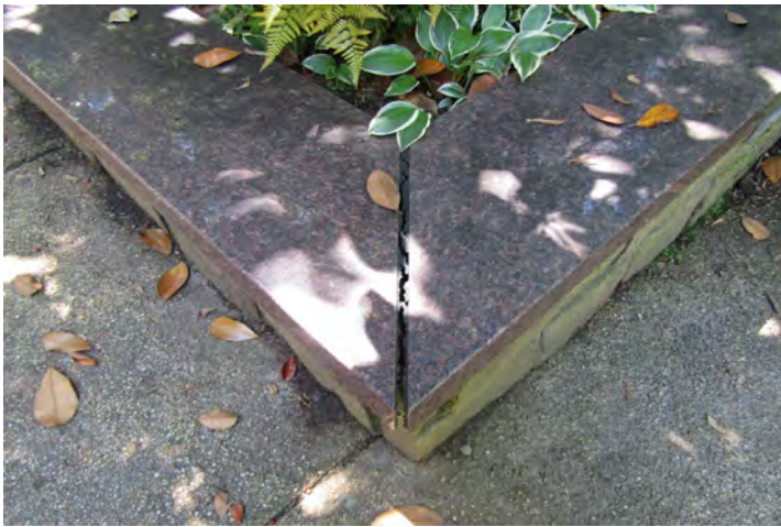
Masonry has shifted
