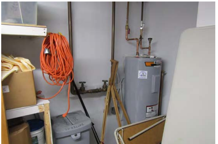
Blocked access to the hot water heater
