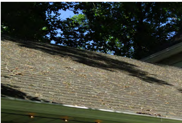
Roof is at or near service life
