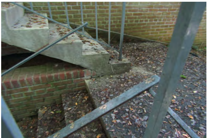
Metal railings are chipped
