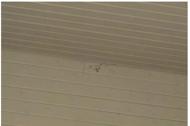
Debris buildup in the high spots
