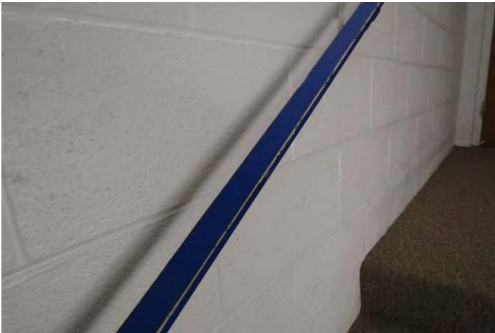
Chipped paint on the handrail
