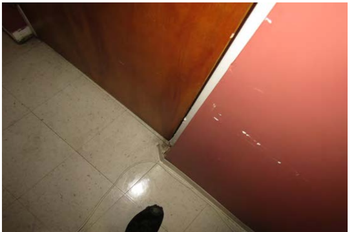
Chipped paint on the wall
