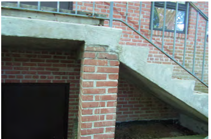
Exit steps need cleaning and repair
