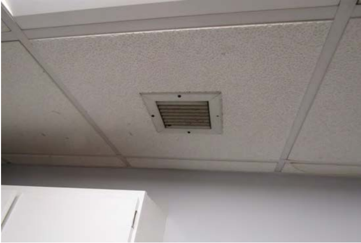
Debris buildup on the exhaust vent
