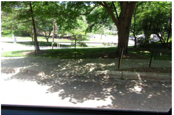
Curb cut is not well marked
