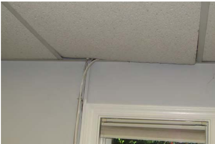
Improper cable access through the ceiling tile
