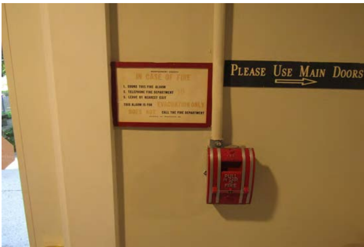
Unmonitored fire alarm
