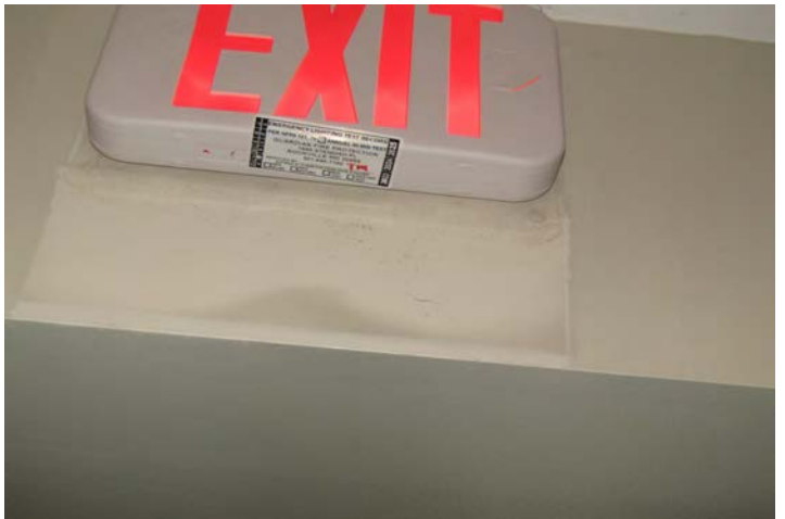
Wall touchup needed
