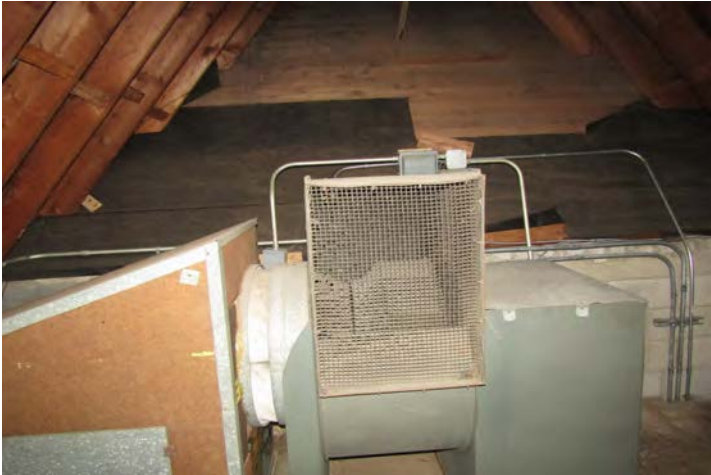
Air exchanger over the Montessori School entrance
