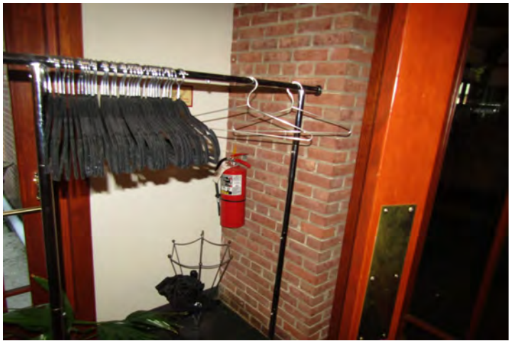
Blocked access to the fire extinguisher and door
