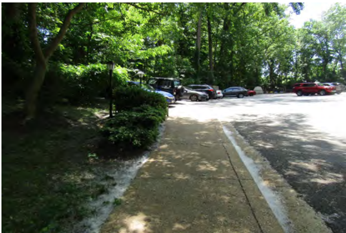
Sidewalk needs safety bollards and handrails
