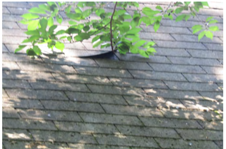
Tree branch growing in the shingles
