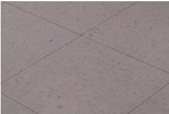
The VCT needs a strip and re-wax
