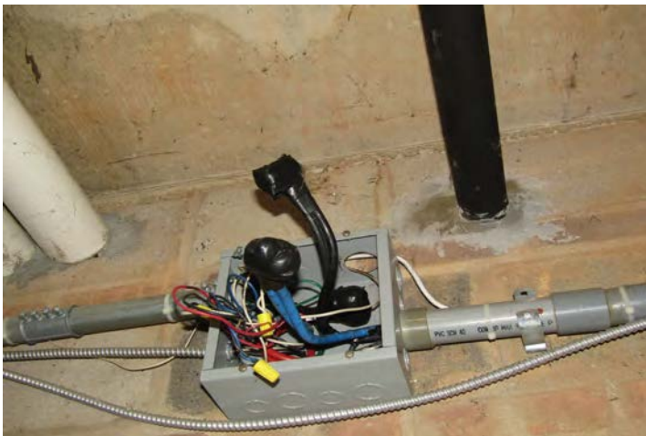
Improper electrical connection, missing junction box cover
