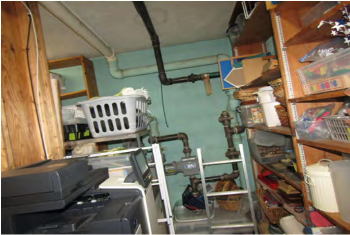
Gas main access is blocked
