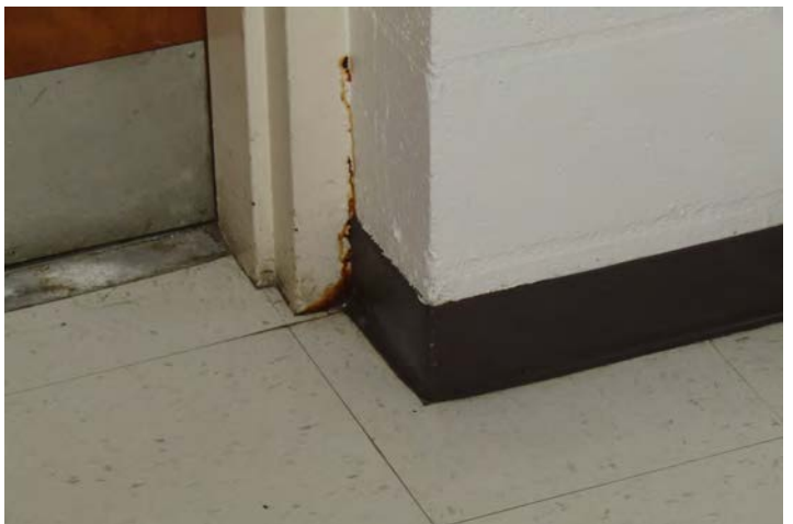
Rust and staining on the door frame
