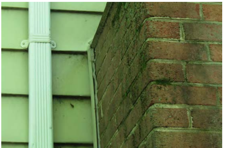
Organic buildup on the brick
