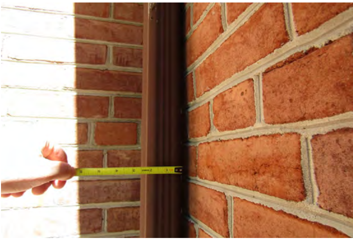
Downspout size is too small for volume
