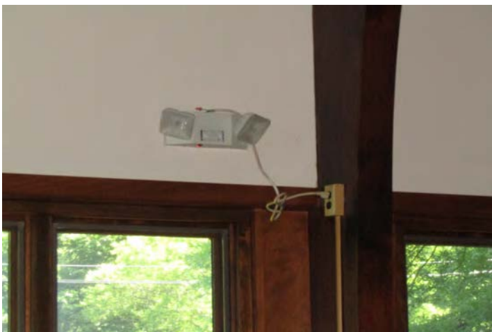
Incorrectly wired emergency exit light
