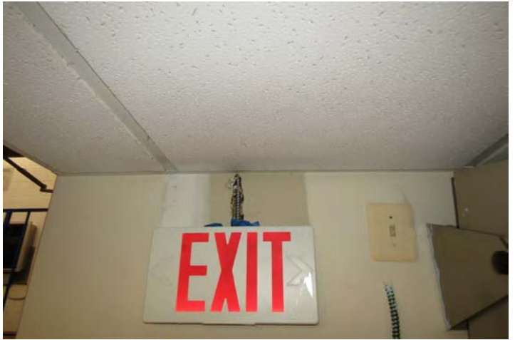
Improper MC8 installation and wall needs touchup
