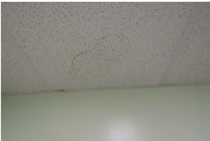
Stained ceiling tile
