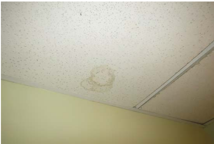
Stained ceiling tile
