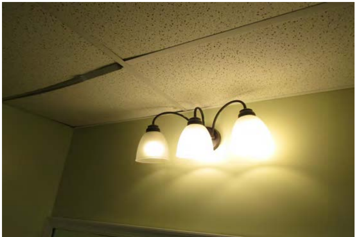
Ceiling tiles out of place
