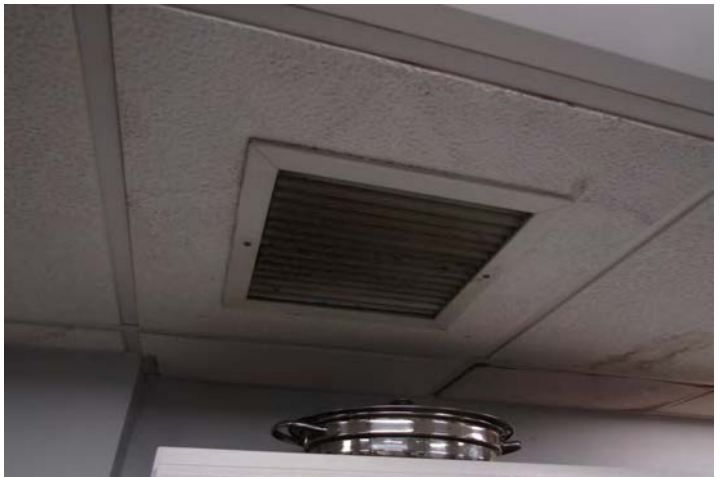
Debris buildup on the exhaust vent
