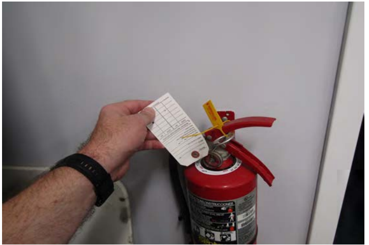
Monthly inspections are not noted
