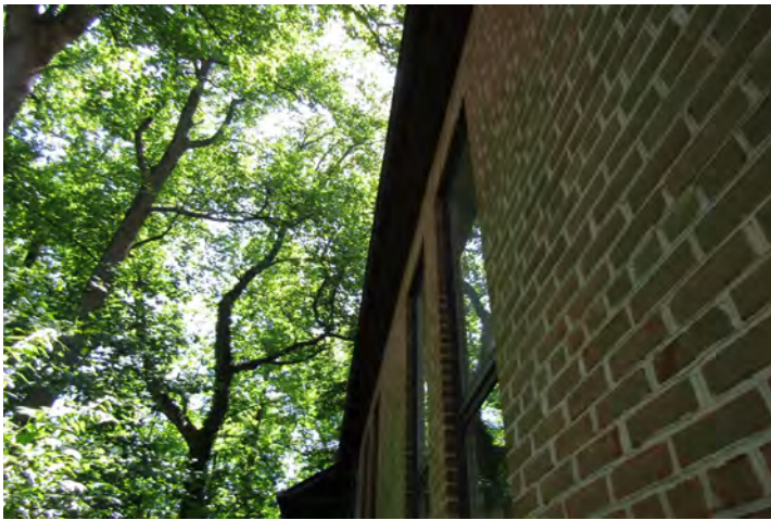
Trees are growing too close to the building
