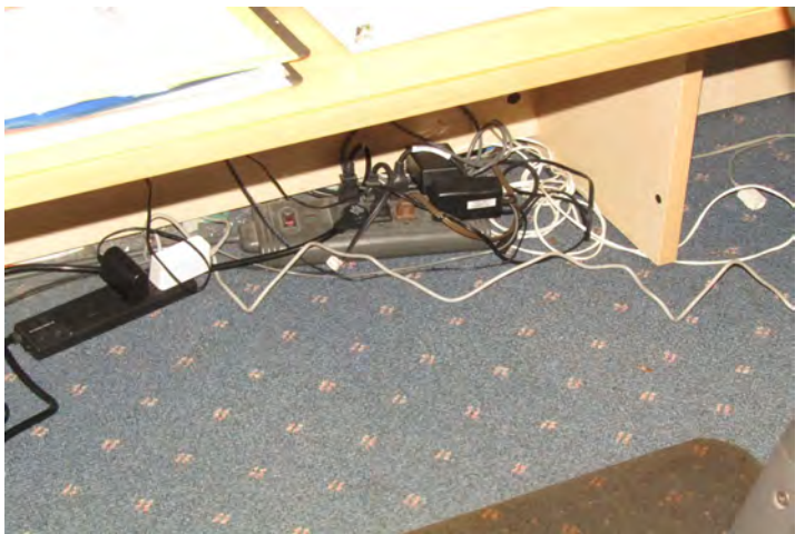
Unsafe cable management
