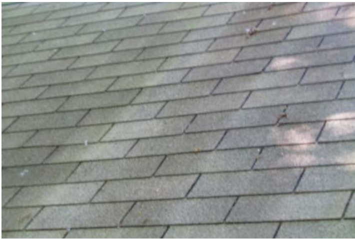
Shingles are past service life
