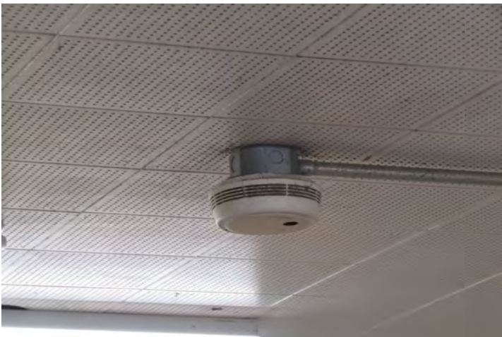
Debris buildup on the sensor
