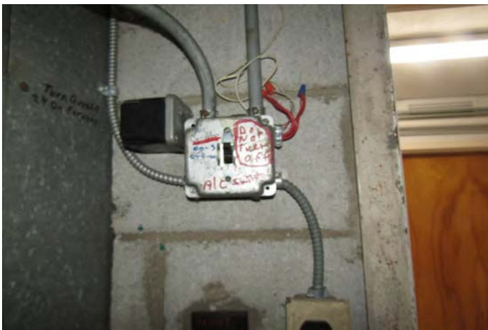
Improperly contained wires
